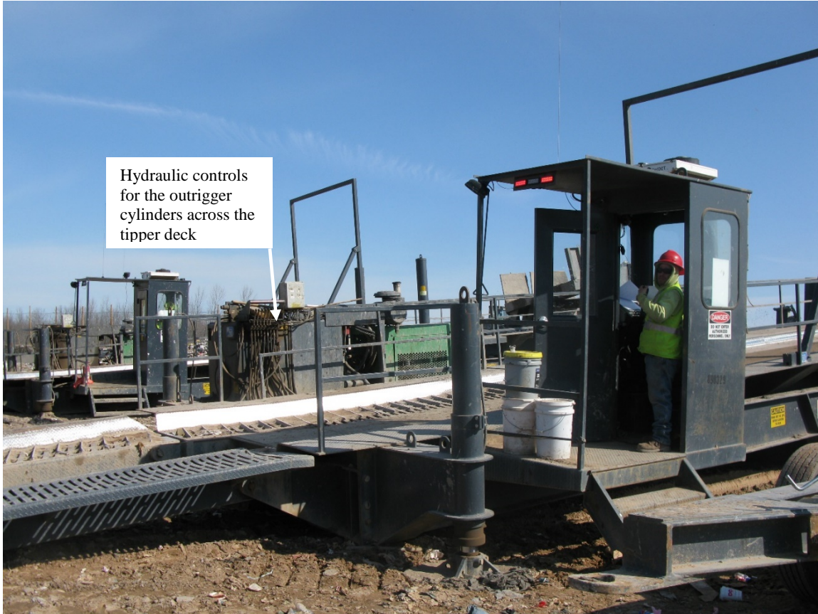
Photo 2. Hydraulic controls for the outrigger cylinders were on the left side of the deck and the operator's cab was on the right side.
