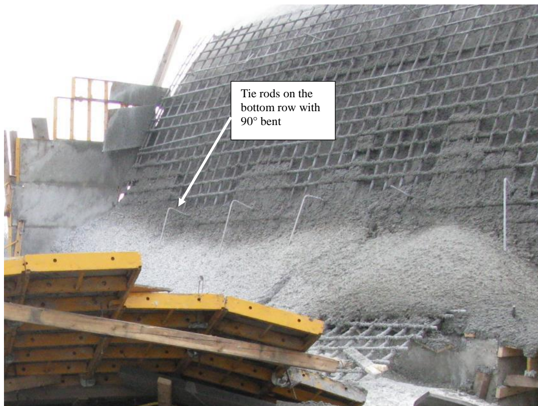
Photo 4. Tie rods that remained on the concrete bent at a nearly 90° angle suggesting a vertical drop in the retaining wall during collapse (photo courtesy of OSHA).
