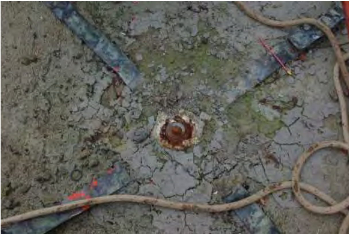
Photo 4. The cement base with a metal pin embedded. The base of the tower was mounted on the pin (photo courtesy of OSHA).
